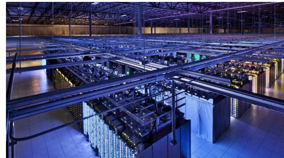
Data Center Cooling
